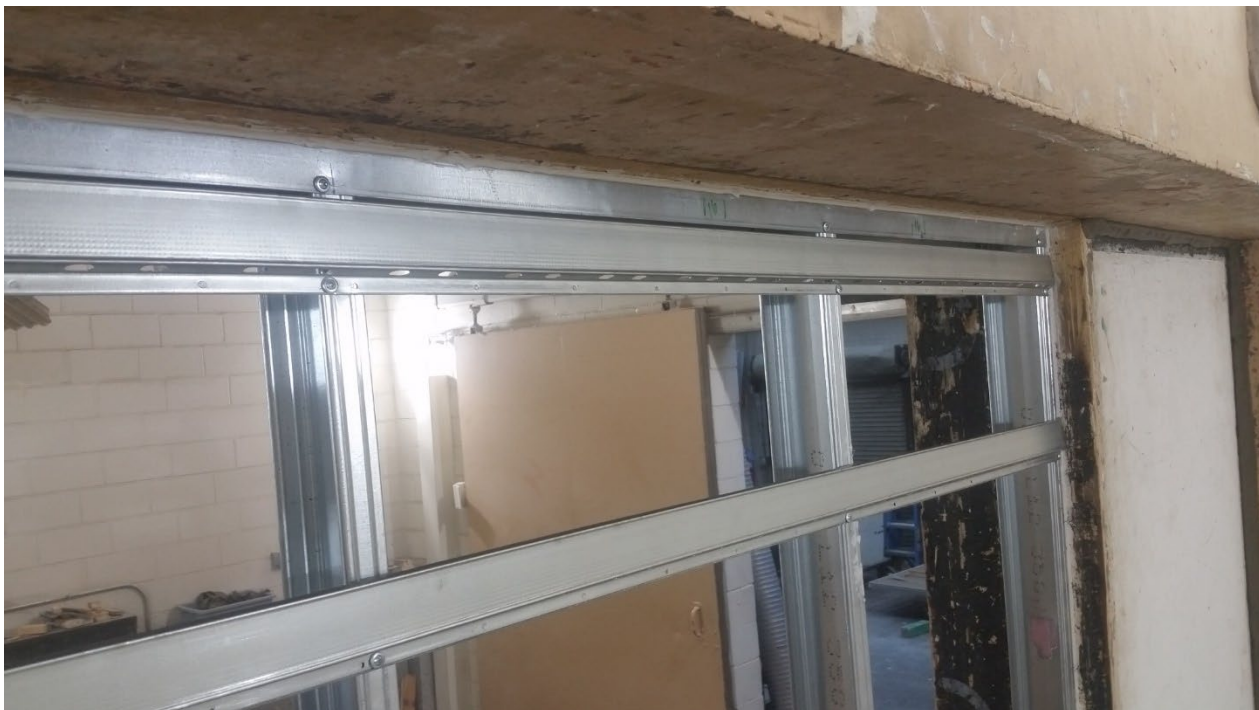
Figure 4 – Detail of studs fastened to track, and resilient channel fastened to studs
