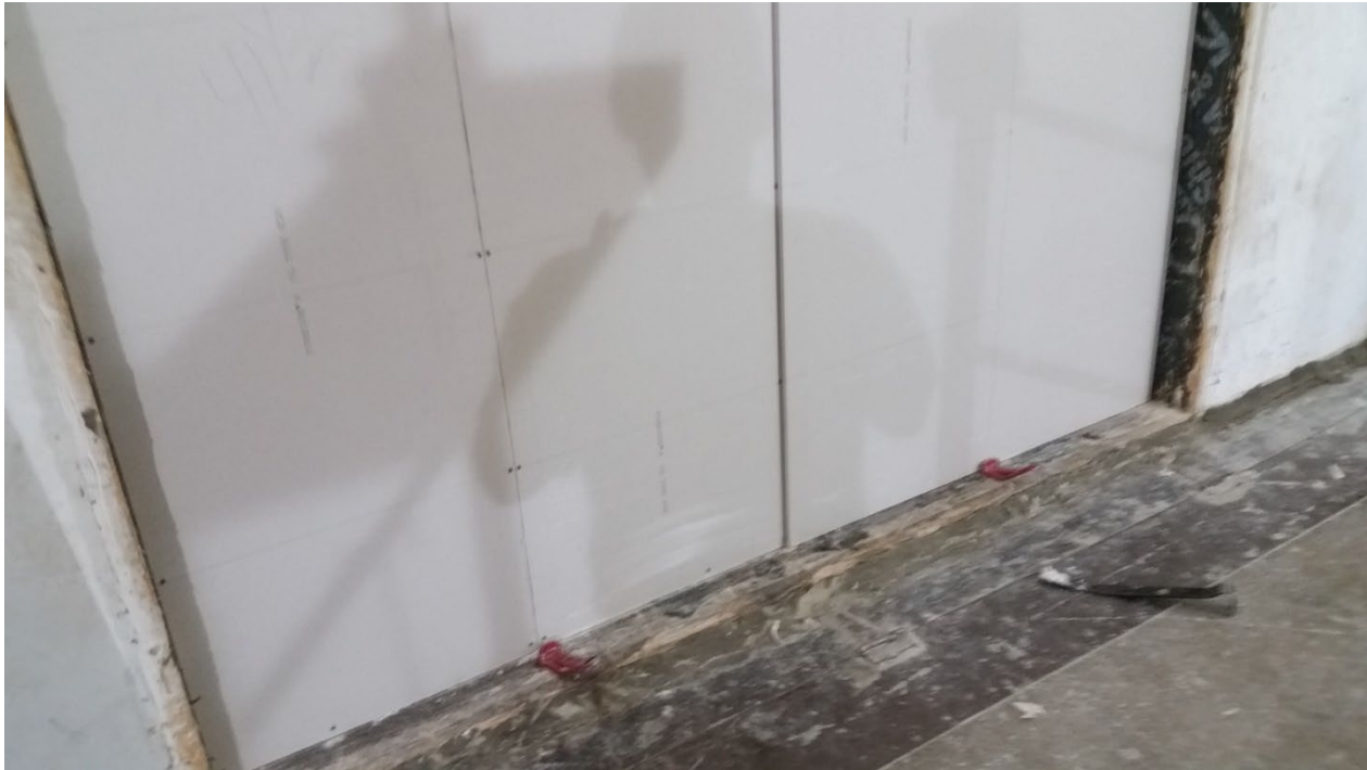
Figure 9 – Receive room side face layer gypsum partially installed, view from receive room
