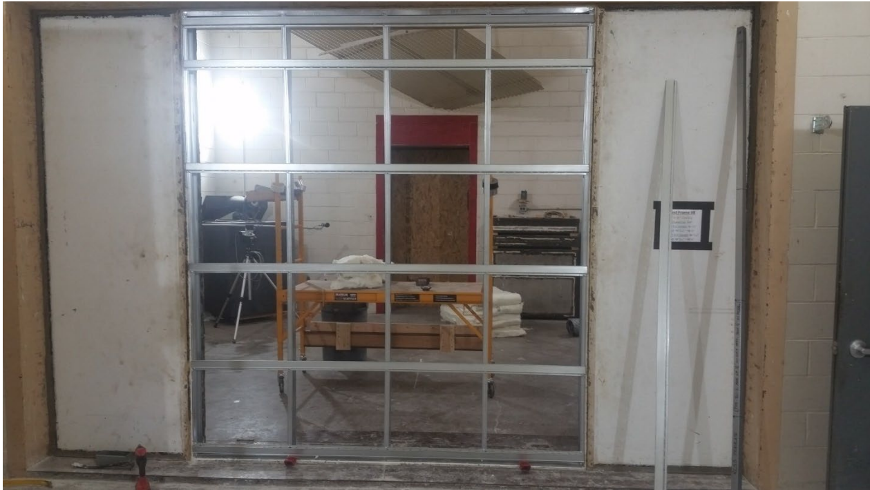
Figure 3 – Tracks, studs, and resilient channel installed in test aperture, view from source room side
