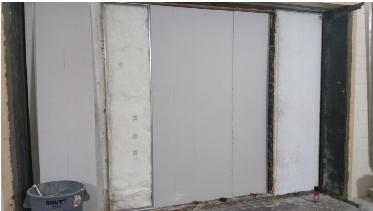
Figure 8 – Receive room side base layer gypsum partially installed, view from receive room
