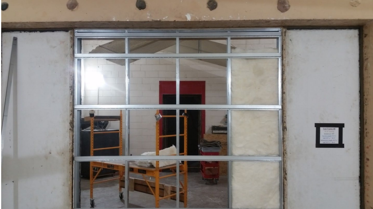
Figure 3 – Tracks, studs, and resilient channel installed in test aperture; insulation partially installed
