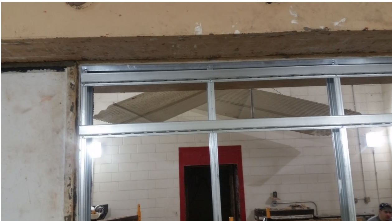
Figure 4 – Detail of resilient channel installed to studs, viewed from source room side
