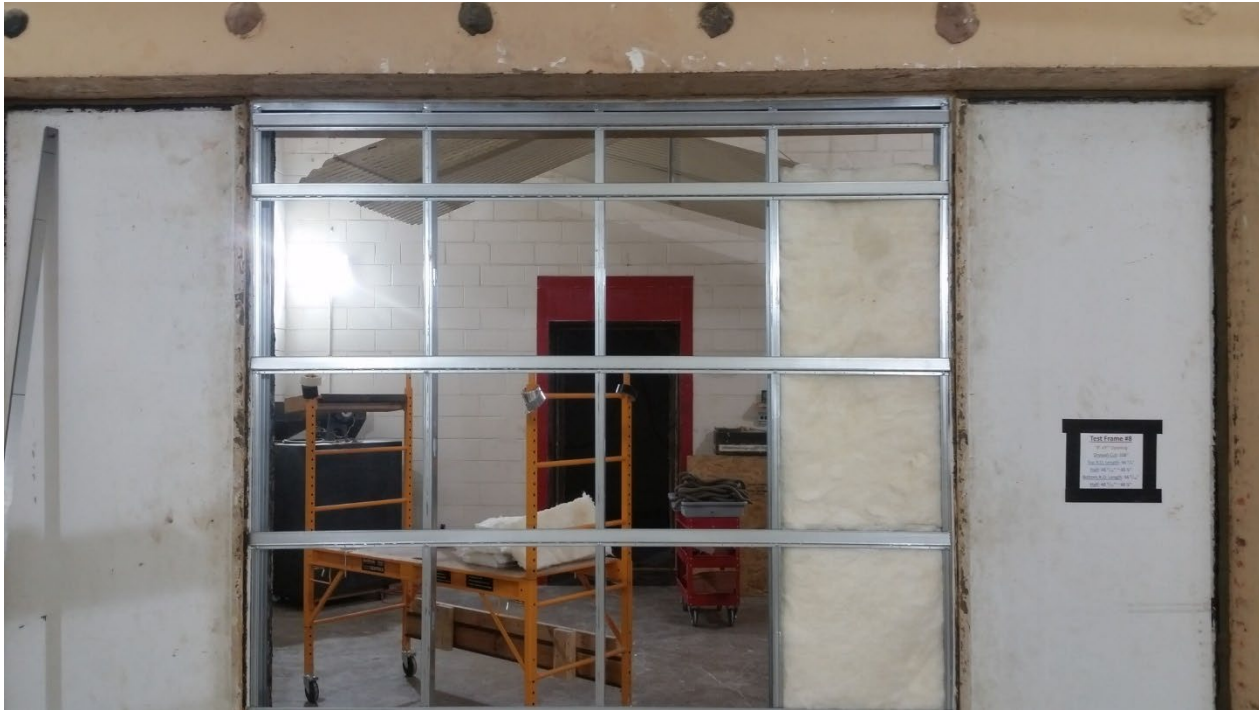
Figure 3 – Tracks, studs, and resilient channel installed in test aperture; insulation partially installed
