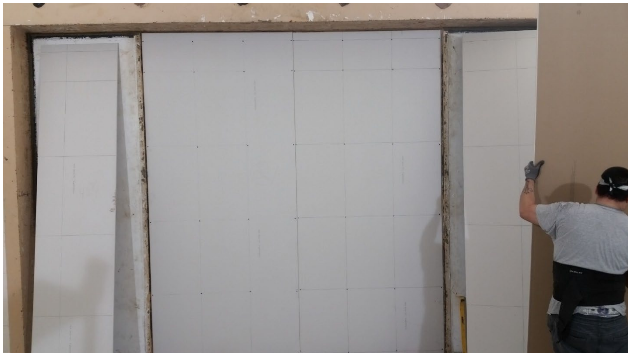
Figure 6 – Base layer of source room side gypsum board installed, as viewed from source room
