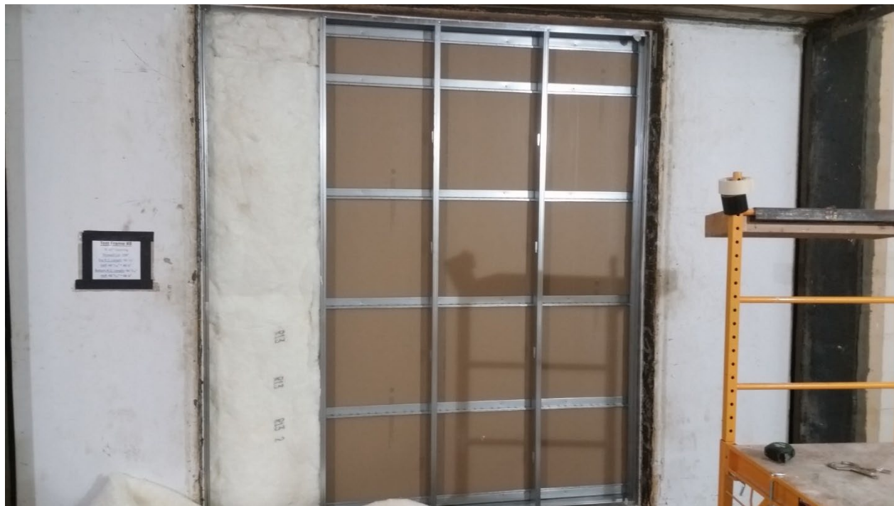
Figure 7 – Source room side gypsum installed, insulation partially installed, viewed from receive room side
