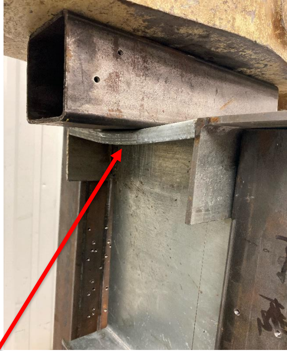
YIELDING OF TOP FLANGE
